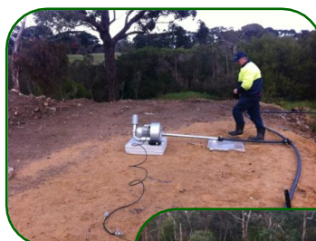
These 3 pictures show the aeration system being installed, and then in working order.
